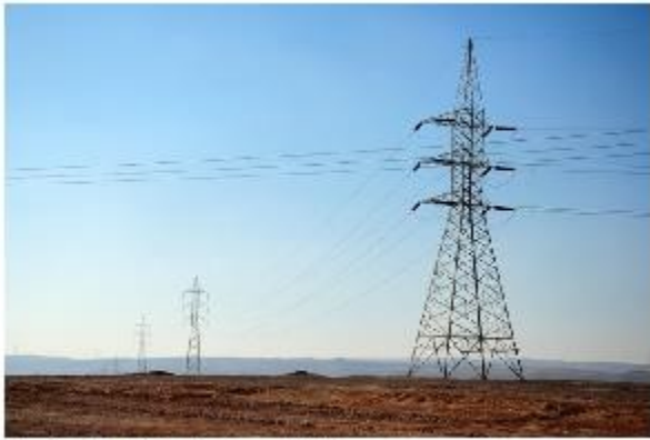
Jordan Electricity Sectors - Plant
