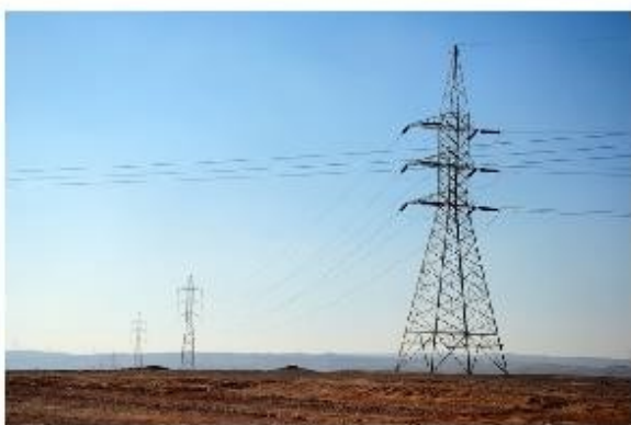
Jordan Electricity Sectors - Plant
